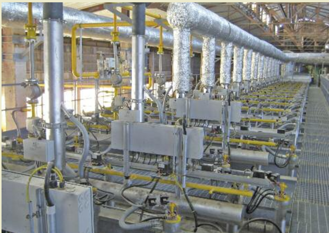
Tunnel kiln with top firing by gas burners
