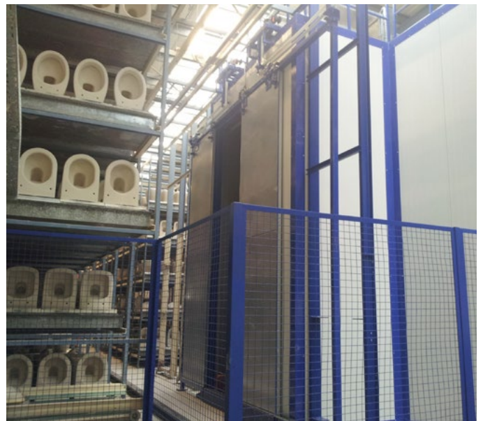
干燥机出口及产品储存 Dryer exit and product storage
