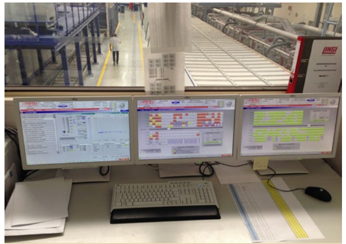
Trocknerleitsystem Dryer control system
